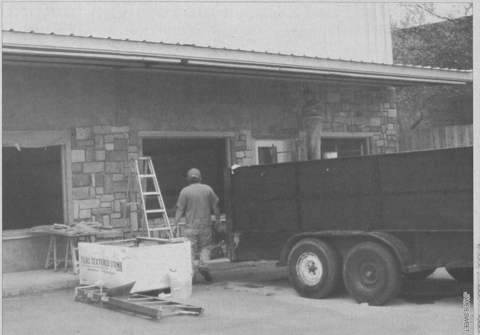
Work continues on the new building on the 300 Block of E. Main Street as workers put stone on the facade.
